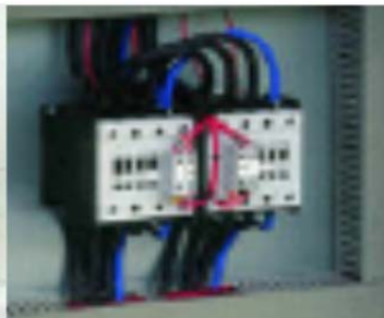
LTS 20-110 (CONTACTORS VIEW)
