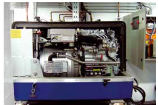
This three-phase Panda is installed in the basement. Main fuses, panel and radiator control are fitted in electrical cabinet. Image: Kratos Kft. Hungary.
