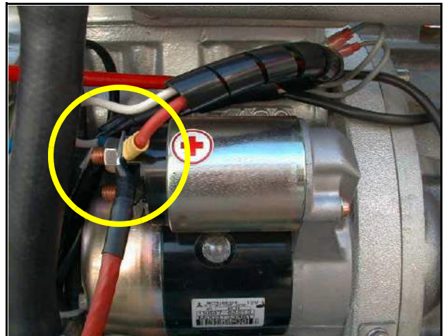
Fig. 5.6.1-1: Positive battery cable
